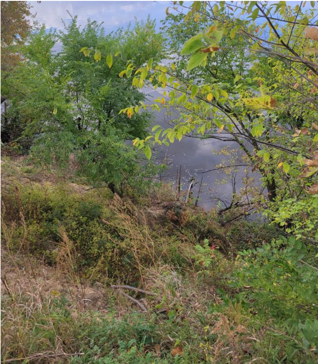
Bluff sloughing behind Lot 7 from top of bluff
